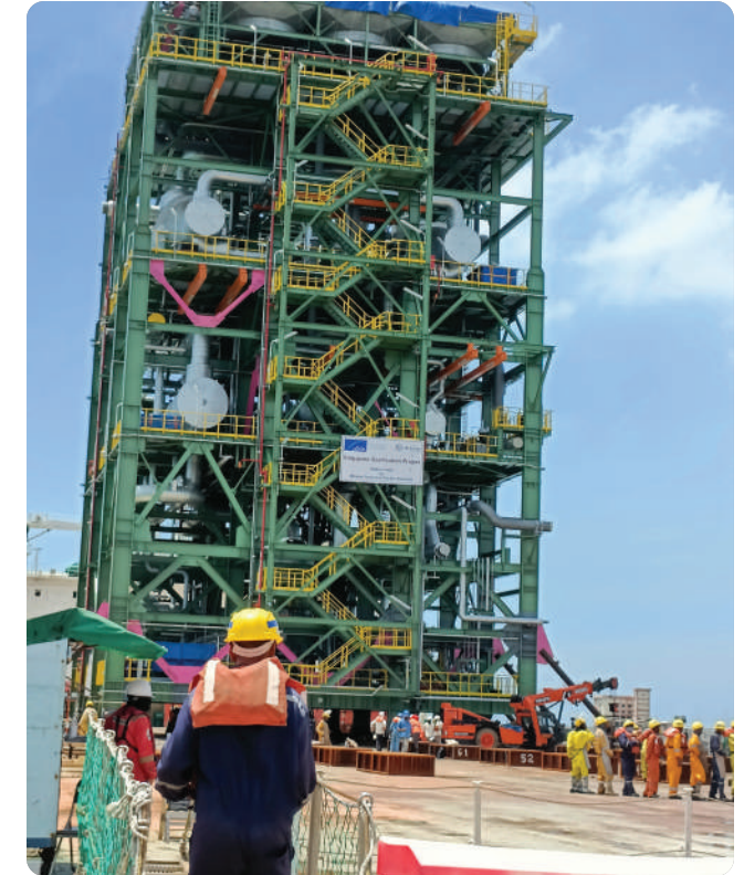
Linde New Gasification Plant Project at Kattuppalli Chennai by Asian Paints PPG (Contractor - L&T Energy Hydrocarbon)
